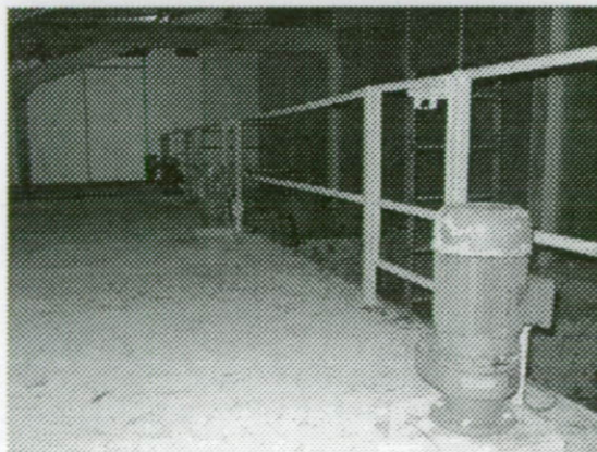
CENTRAL BYPRODUCTS STORAGE IN CONCRETE PITS WITH MIXING-UNITS
