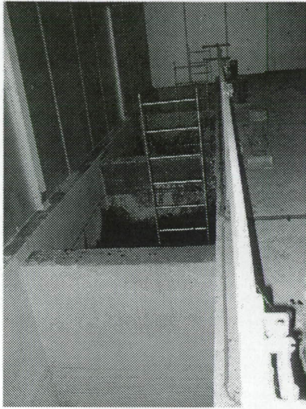
PITS FOR BYPRODUCTS WITH STAINLESS STEEL ACCESS LADDER
